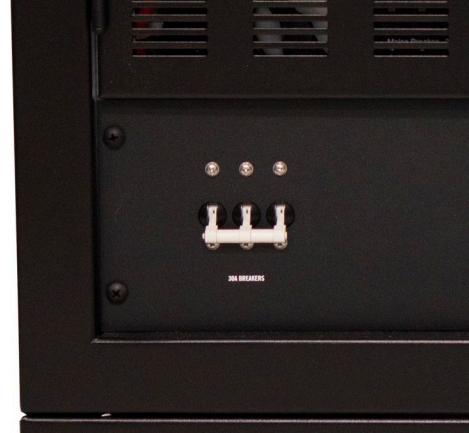
Figure 7.2 Main Power Breaker Switch
